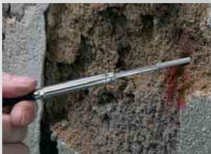
Inserting the humidity probe in a bore hole with PTFE protective cap
